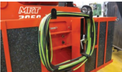
Grounding by rod
